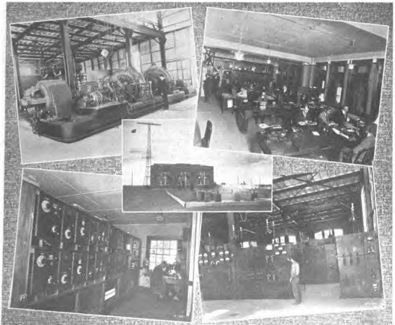
Radio Central Power House and Cooling Pond in the Center. High Frequency Alternators on Upper Left. Receiver Section on Lower Left. Operating Room on Upper Right, and Main Switchboards on Lower Right.
